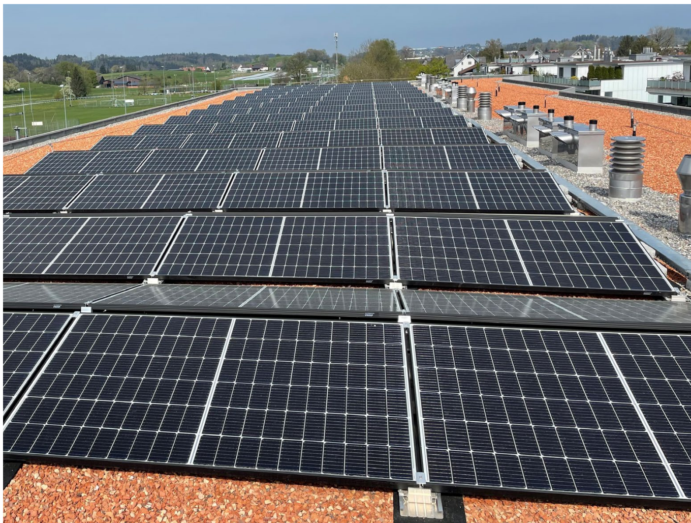
Fehraltorf (ZH), Wermatswilerstrasse 20: Installation photovoltaïque
